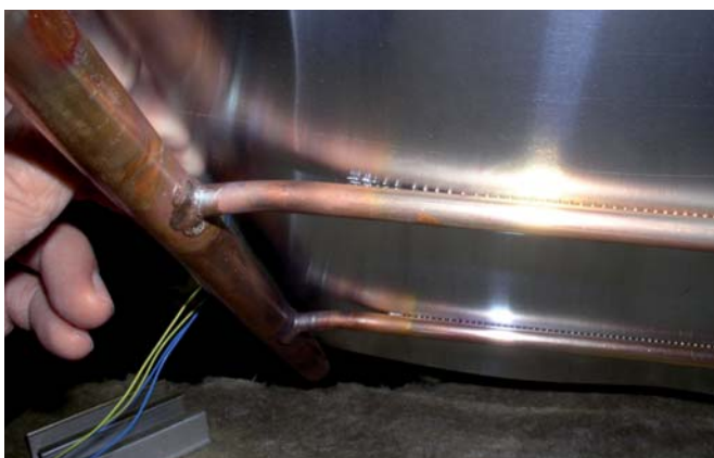
Figure 14: Mild separation of one of the ascending pipes.
